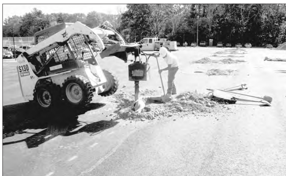
A Bobcat drills spots for the net posts at the new tennis courts at Andover High School.
