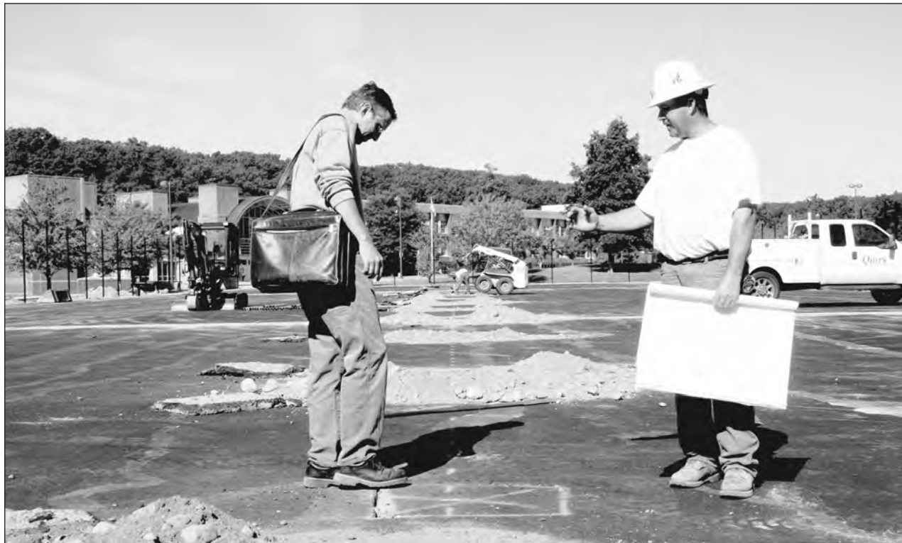
Project architect Chris Huntress of Huntress Associates looks over the tennis court site with Quirk Construction Corp. foreman Mario Moura.
