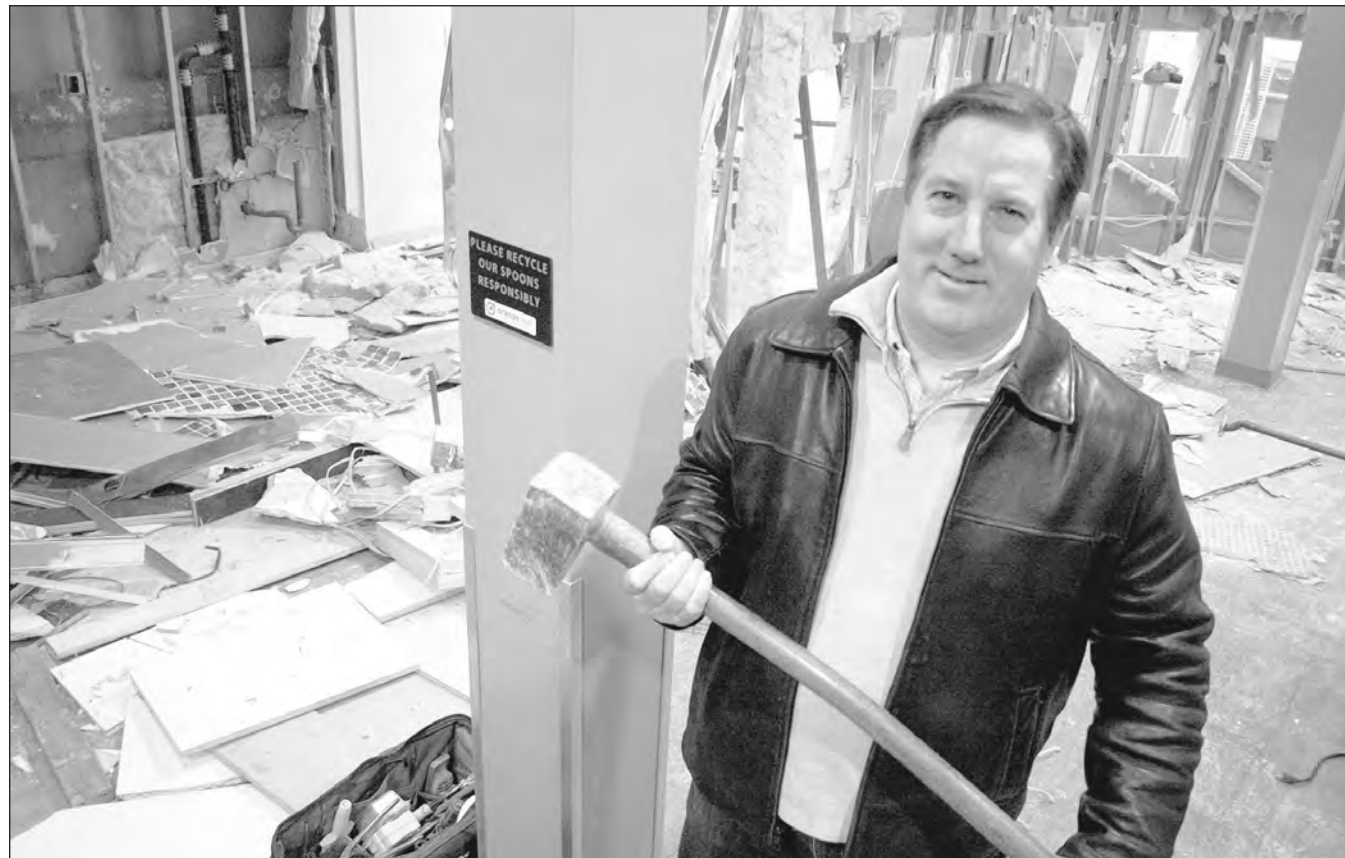
Dave Pierre, owner of four Orange Leaf franchises, is in the midst of a major renovation and expansion of his original Park Street location in downtown Andover. He is hoping to unveil the new space during a grand re-opening on Feb. 14.
