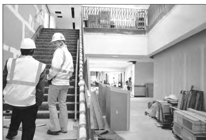
Dennis Forgue, who recently stepped down as chairman of the School Committee, walks up the main stairway to the second floor of the new Bancroft School last month with a representative of the developer, Skanska. In the background, contractors work in the school's main, first-floor hall, which leads to the kindergarten and first-grade wings.
