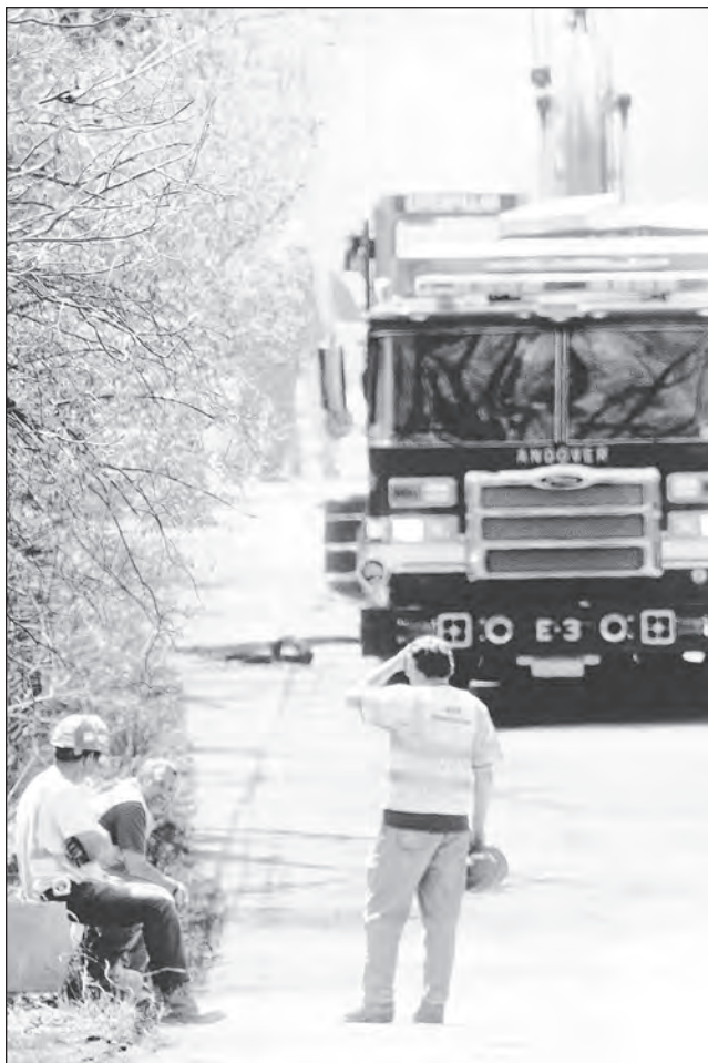
PAUL BILODEAU/Staff photo A construction crew stands back after a gas main was ruptured on River Road near Cross Street in Andover last Thursday afternoon.
