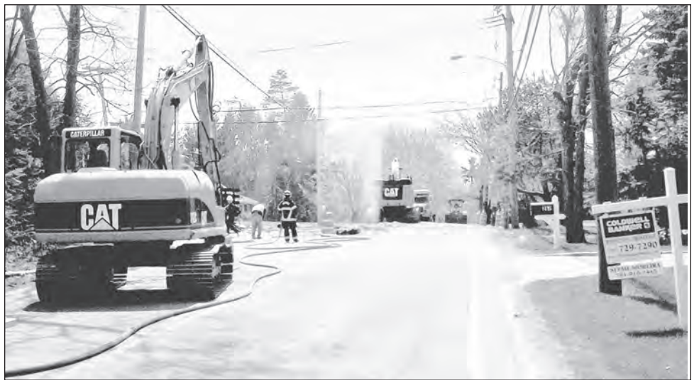
BILL KIRK PHOTO A gas leak on River Road near the intersection with Cross Street created a geyser that rose into the air about 20 feet from a trench in the road. The geyser is faintly visible near the Caterpillar excavator, on the right, in this photo.
