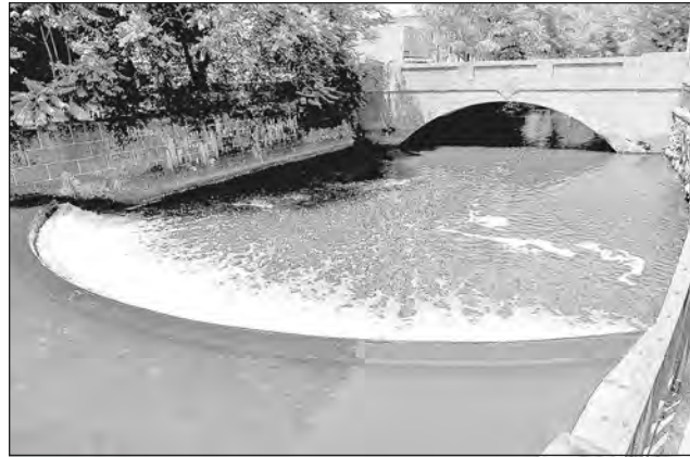
The Shawsheen River dam next to Balmoral Condominiums in Andover is slated to be removed as early as next year.
