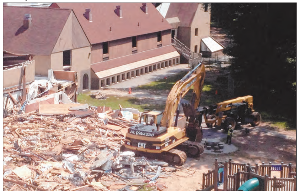
Demolition crews began taking down the old Bancroft Elementary School section by section on Tuesday. The building is expected to be fully leveled by early next week.
