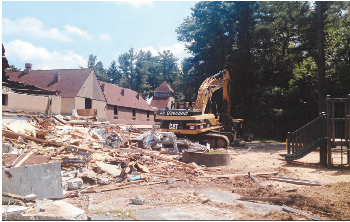
A construction vehicle works to gather debris torn off the old Bancroft Elementary School on Tuesday. For more photos of the demolition, see page 8.
