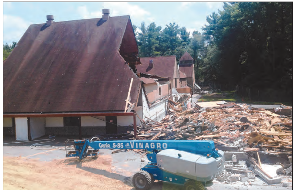
A section of the old school is reduced to rubble after the first day of demolition on Tuesday.
