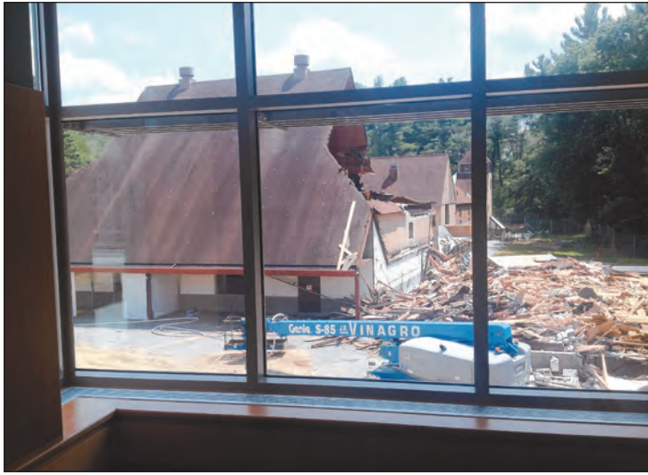
The image of a giant hole torn into what was once the Bancroft gymnasium as seen from the second floor of the new Bancroft Elementary School.
