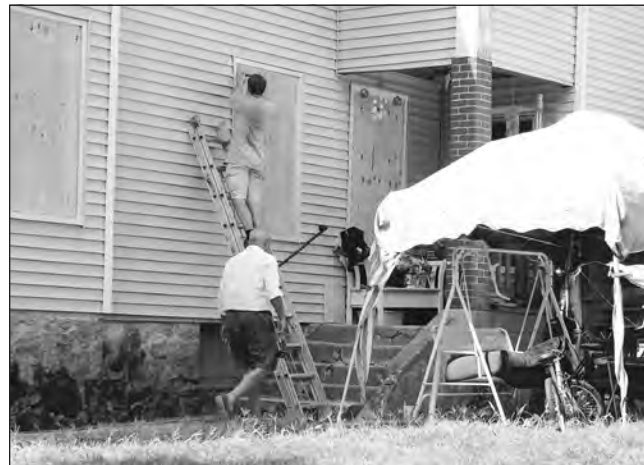
A worker on Tuesday boards up a window on the first floor of 2-4 Duffton Road.
