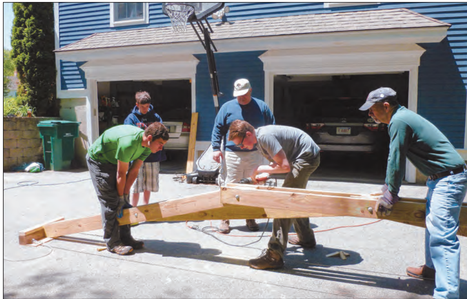
Jeffrey Page works with his volunteer team to construct one of the three trusses to support the footbridge and the footing forms. For more photos, visit us online at andovertownsman.com .
