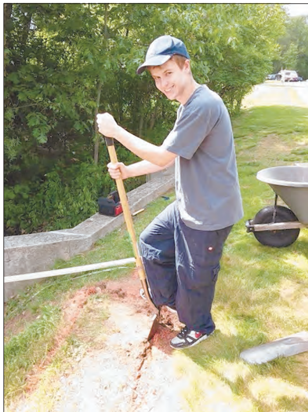
Jeffrey Page digs into the soil as he prepares to set the footing forms in place.
