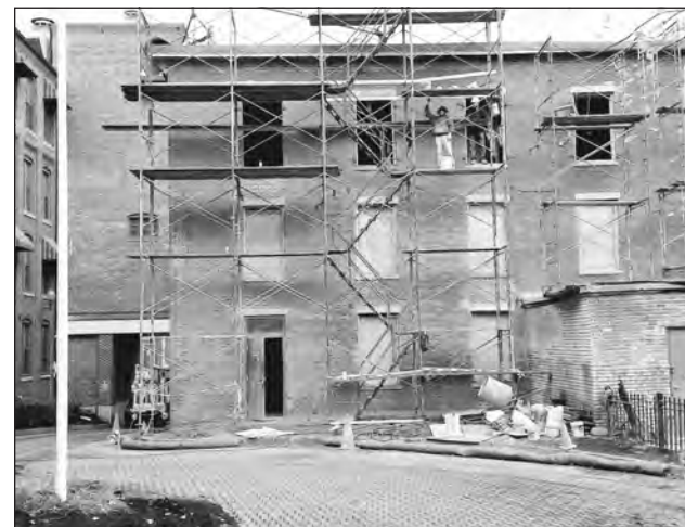
The old mill adjacent to Atria Marland Place on Stevens Street is being renovated to allow for expansion of the senior housing campus.
