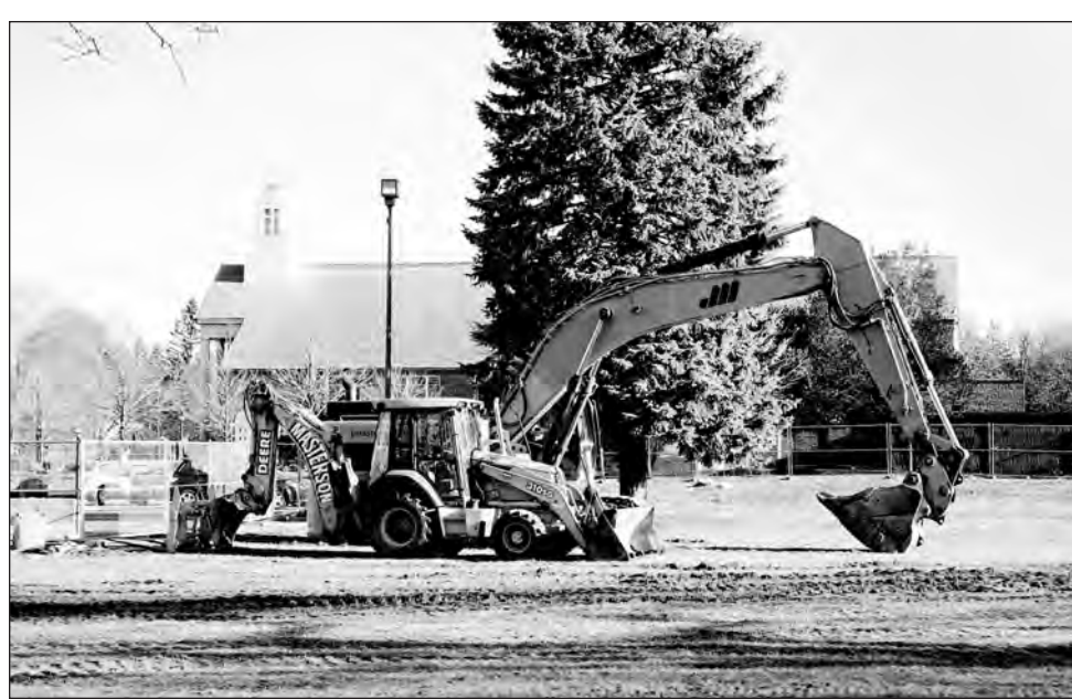
After a lengthy review process, Merrimack College has begun building new dorms and a common building on Austin Field on the college's campus. Construction has begun on the North Andover portion of the site, with final approval still needed for the Andover segment of the project to advance.
