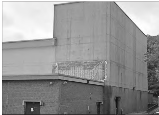
A section of the J. Everett Collins Center exterior wall fell from the building during a storm on Sunday afternoon. The damage is said to be caused by long-term water damage. The road adjacent to the Collins Center will be temporarily limited to traffic, however, except in case of emergency.
