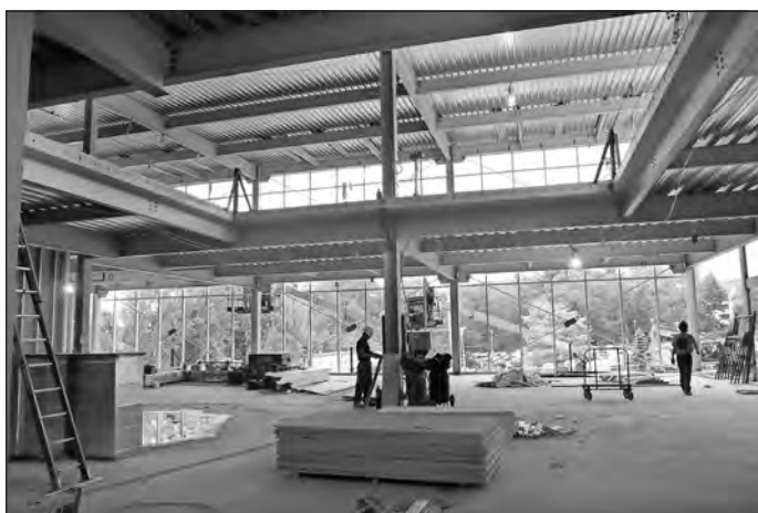
Workers tackle the grand stairway area of the Andover/North Andover YMCA expansion project earlier this month.
