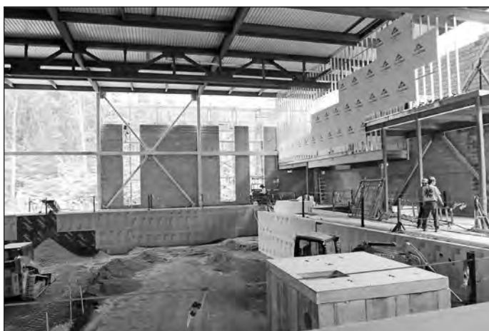
Work continues on the pool area of the Andover/North Andover YMCA branch. The $21 million renovation project includes an expanded aquatics facility with a multipurpose pool.
