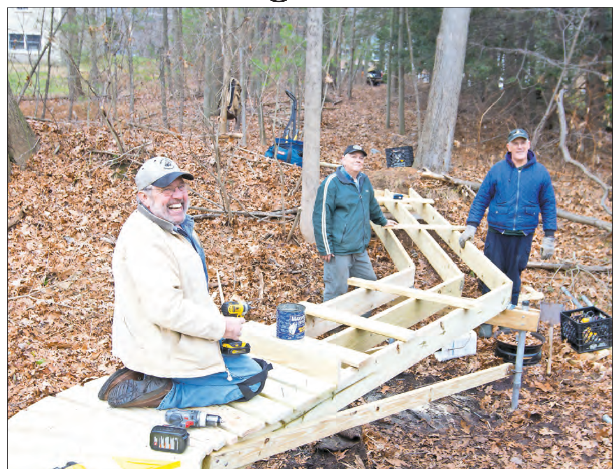
AMY SWEENEY/Staff photo Jim Reilly, left, Bob Decelle and Steve Cooper finish up the boardwalk they have been building on the Bay Circuit Trail located off Serenity Lane in Andover.
