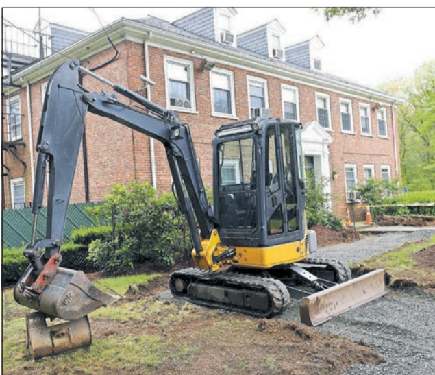
The Andover State Police barracks, originally built in 1920, is currently under renovation. TIM JEAN/Staff photo
