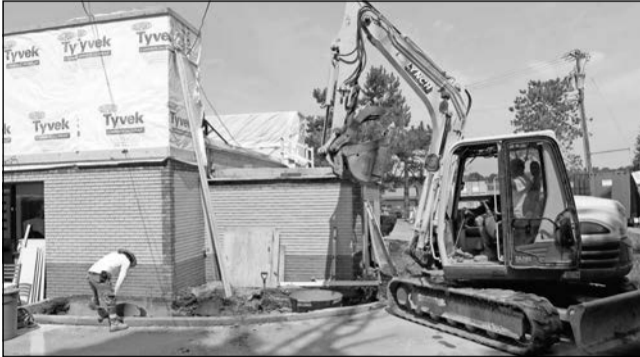
Construction workers use heavy equipment to move gravel while they pour concrete for the footings for the new drive thru.
