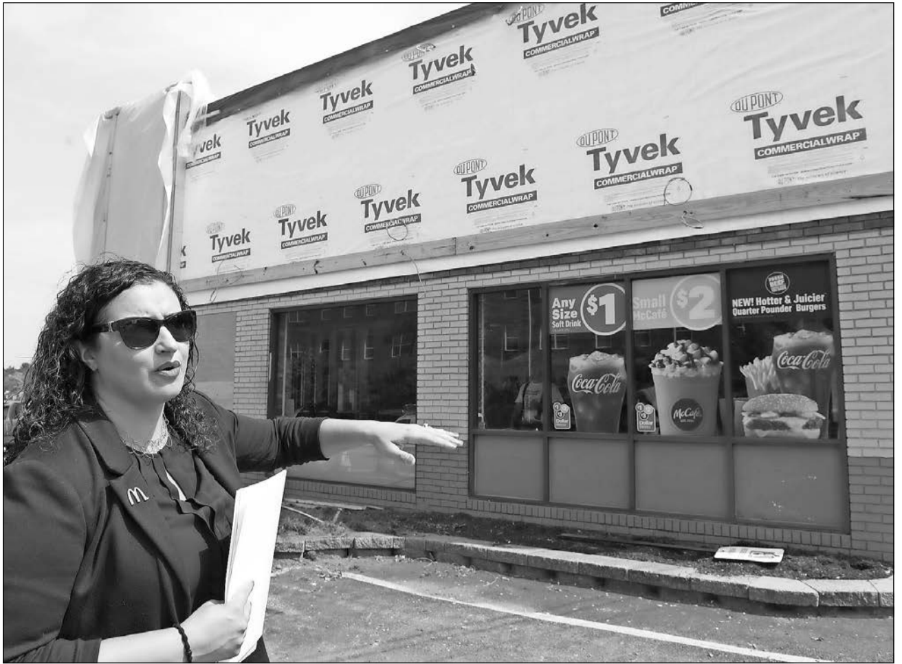
Carissa Haley, owner of McDonald's restaurant in Andover, talks about the new entrances being rebuilt and the improvements being done throughout the restaurant while it's closed for remodeling.
