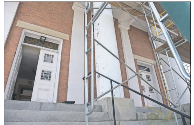
Workers from Painters Pride have installed scaffolding around the Andover Baptist Church entrance to get up to the steeple for repairs and repainting of the structure.
