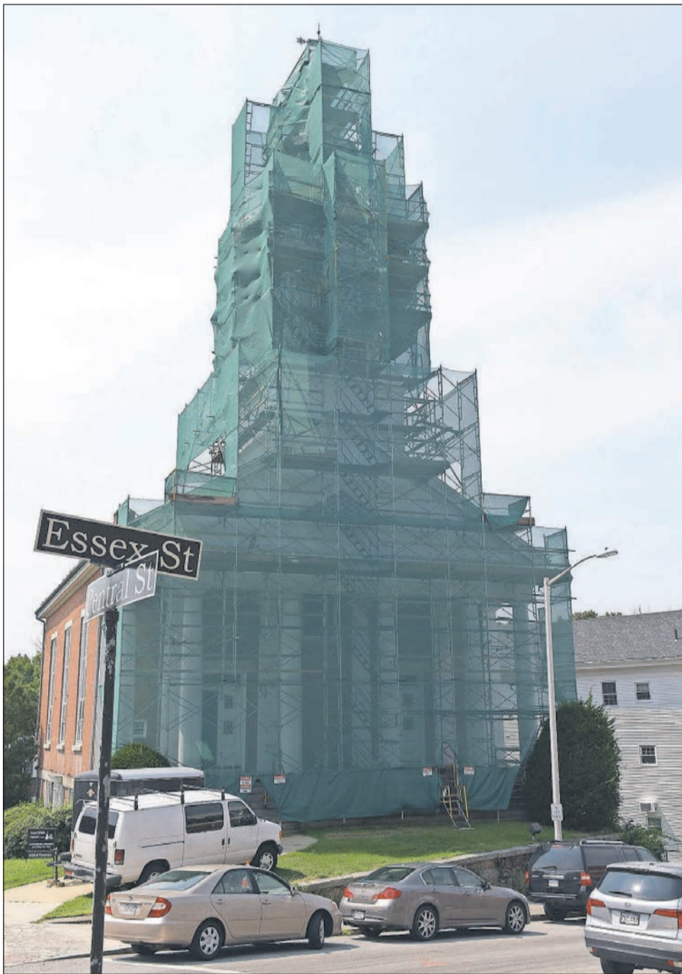
Workers from Painters Pride have installed scaffolding around the Andover Baptist Church steeple while they repair and repaint the structure in downtown Andover.
