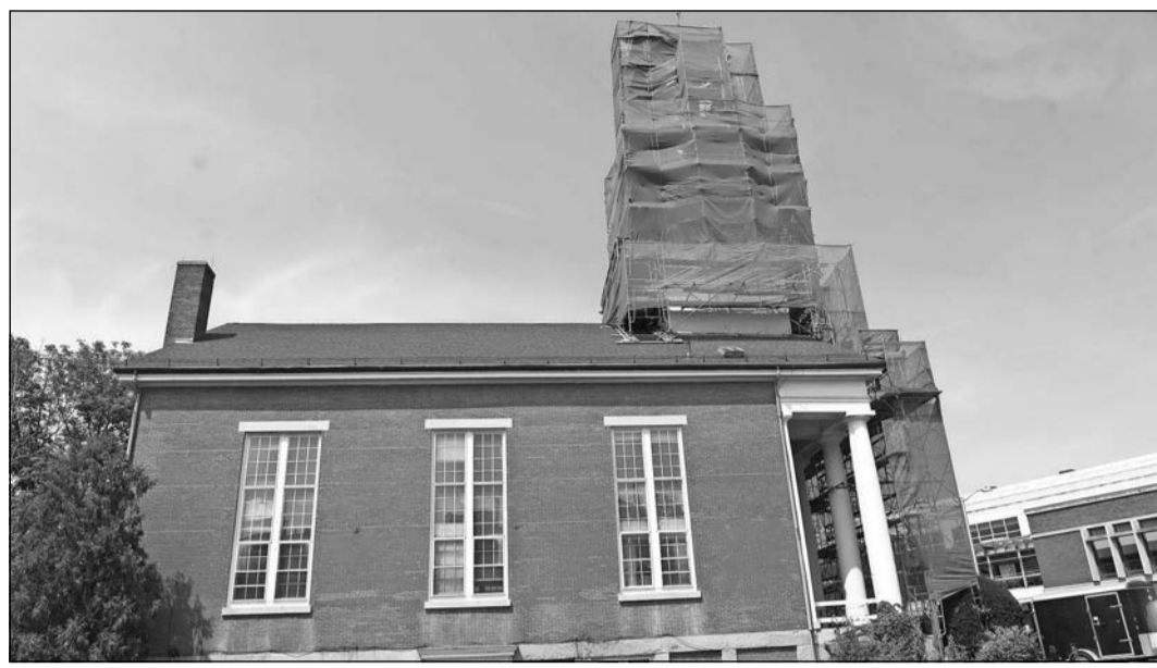
Workers from Painters Pride have installed scaffolding around the Andover Baptist Church steeple while they repair and repaint the structure on Central Street in downtown Andover.
