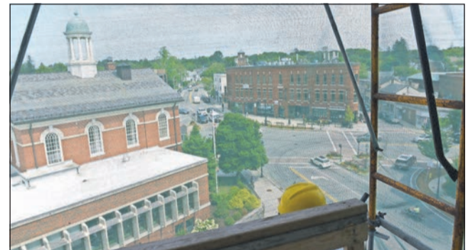
Looking out from inside the scaffolding toward Memorial Hall Library and downtown Andover.
