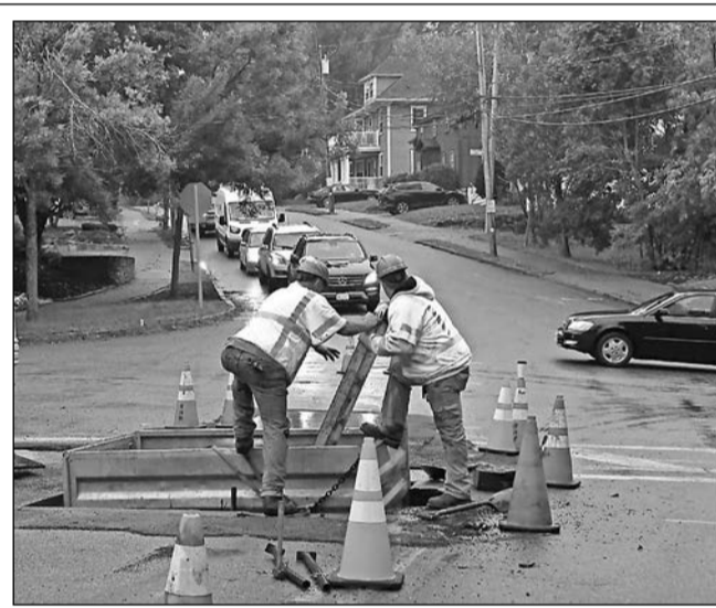
Work crews continue to dig in to the street at the intersection of High and Harding Streets.
