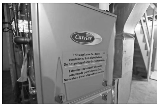
The furnace in the basement of Tom Haynes' childhood home on Mt. Auburn Street has been condemned by Columbia Gas due to damage from the September 13th Merrimack Valley gas disaster.
