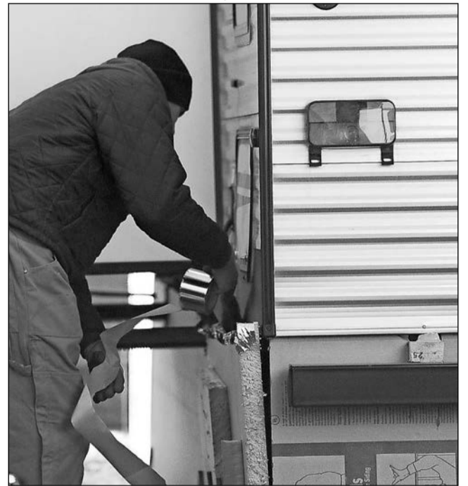
Workers add insulation Saturday to the bottom of a trailer set up for area residents displaced by the Merrimack Valley gas disaster.
