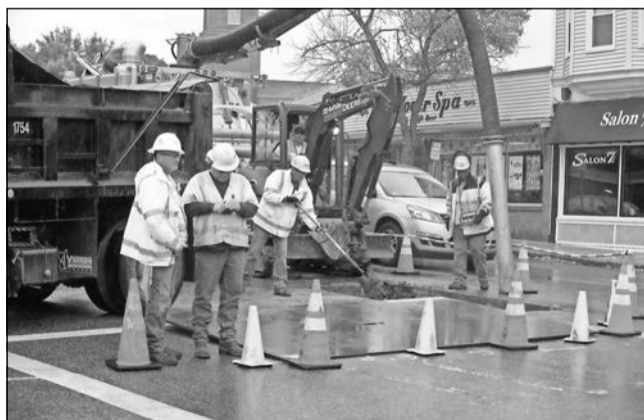
A utility crew from Columbia Gas works at the intersection of Elm and High streets.
