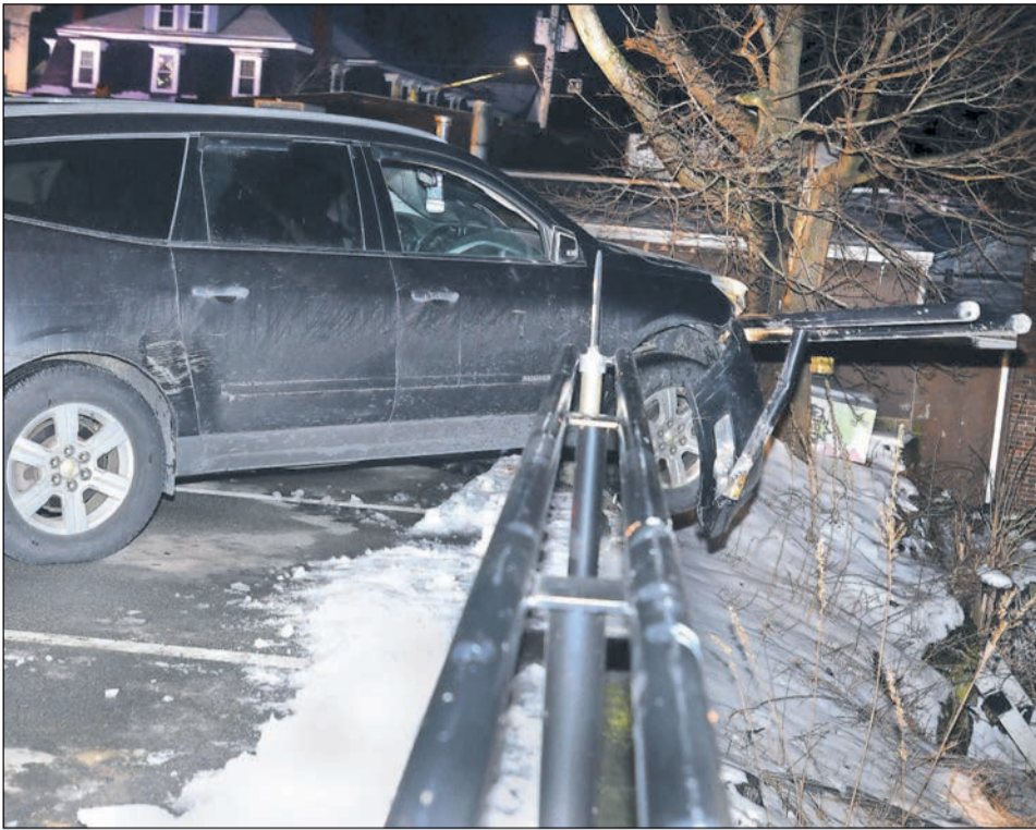
An elderly man avoided serious injury after crashing into a guard rail and wall in the Andover Memorial Hall Library parking lot Thursday night. The vehicle broke through and damaged the guard rail and wall that prevented the vehicle from dropping 20 feet to a parking lot below.
