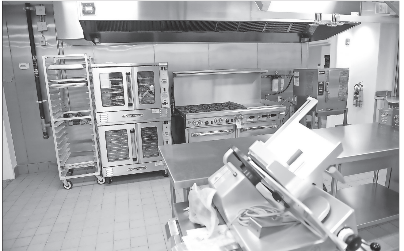
The Robb Senior Center in Andover includes a the new kitchen after a major renovation. The center makes lunch and diners for its meals on wheels program and can serve as an emergency shelter.
